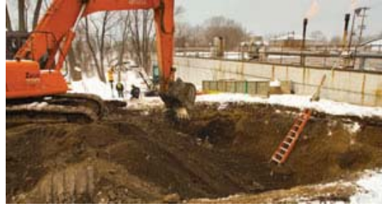
A renewable energy combined heat and power project with City Brewery in La Crosse, Wis., is expected to generate 3 million kWh of electricity per year by using waste methane gas discharged from the brewery's waste treatment process.
