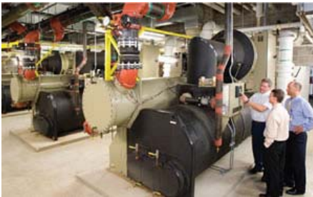
Programs to optimize cooling tower fan utilization with chiller compressors have reduced costs by approximately $65,000 a year and reduced energy consumption by about 1.1 million kWh annually.
