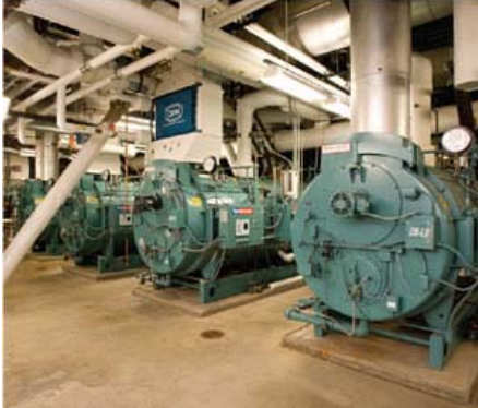
Converting high-pressure steam to low-pressure allows the health system to turn off several boilers in one of its outpatient buildings, saving nearly $64,000 annually.
